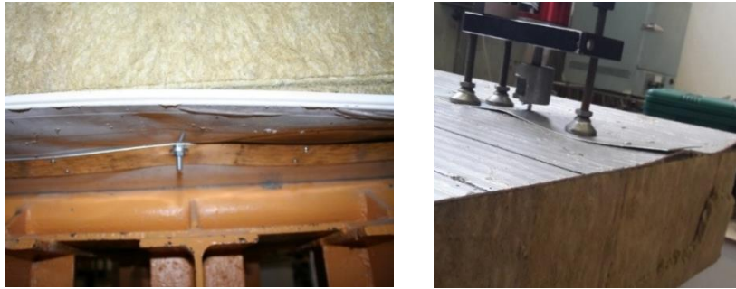
Figures 16 and 17. Delamination of sandwich panel
