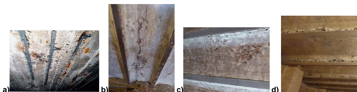
Figure 2. Types of damages in Prussian vaults made from brick aggregate concrete: a – corrosion of steel beams, b – cracks, c, d – degradation of the material
