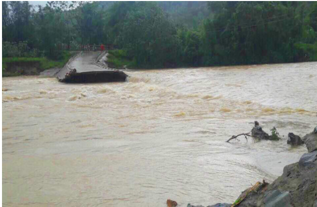
Figure 1. A-Sap bridge collapsed in Thua Thien Hue province, Vietnam, November 2016.
