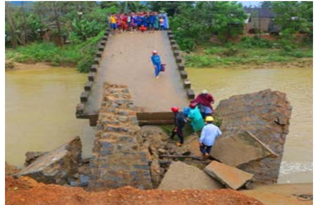
Figure 2. A bridge collapsed in Hoai An, Binh Dinh province, Vietnam, 2016.
