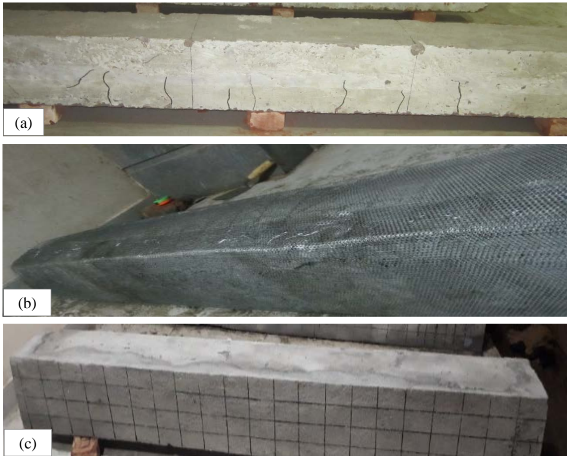
Figure 2. Retrofitting via ferrocement technique: (a) partially damaged beam, (b) the wire-mesh around the partially damaged beam, and (c) retrofitted beam before the flexural test.
