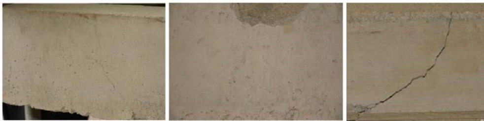
Figure 7. Cracking in the beam with metal reinforcement.
