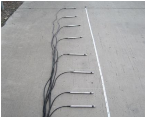
Figure 2. General view of one set of the temperature and moisture sensors.
