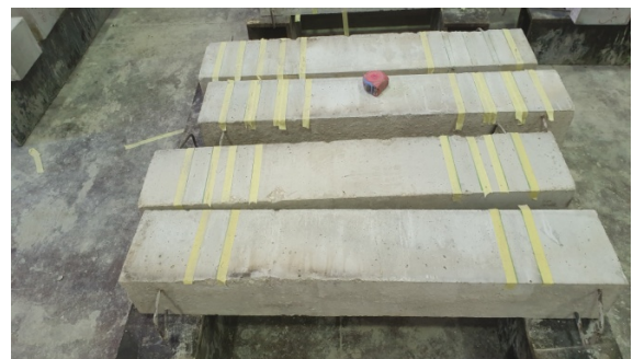
Concrete bonded area were roughened and brushed with steel wire cup brush
