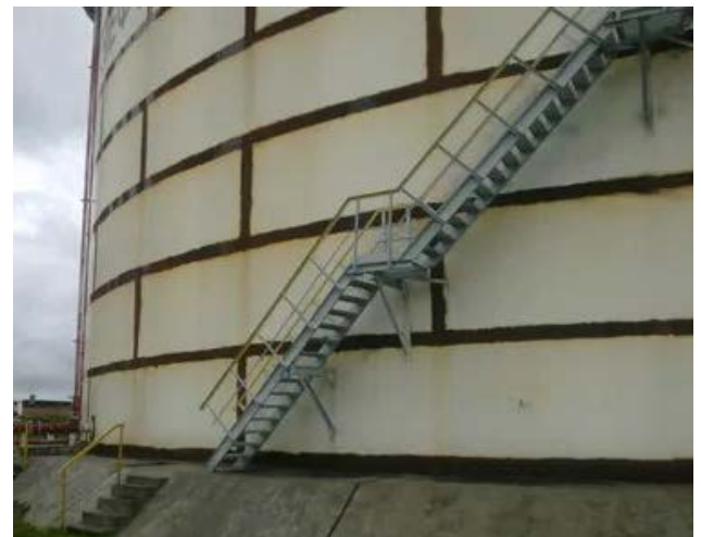
Figure 1b. Spiral tank staircase.
