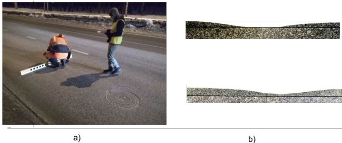
Figure 1. Wear rut investigation in Kazan: (a) rut propagation monitoring by Glavtadortrans; (b) transverse profile of rut by the KGASU [8].
