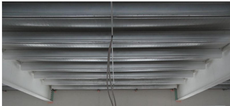
Figure 2. Bottom view of the floor slab of the second floor: significant deflections of the ribs of the profiled steel sheet.
