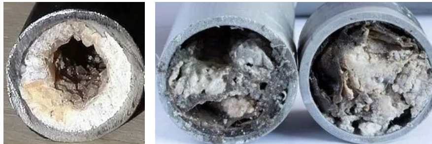
Figure 1. Partially or completely clogged sewer pipes [4–8].
