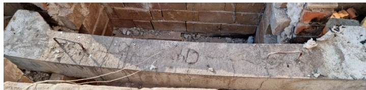
(c) Crack pattern for 750 °C temp. Specimen.
