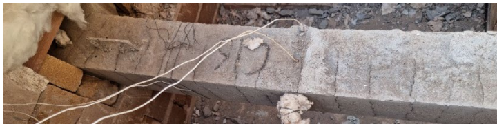
(b) Crack pattern for 600 °C temp. Specimen.
