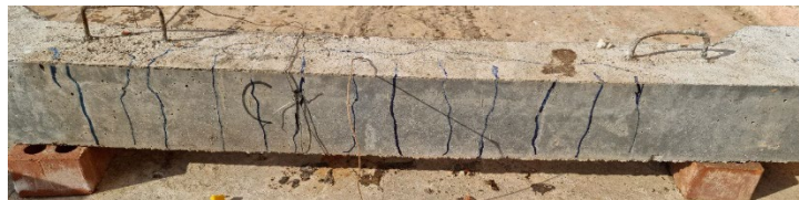
(a) Crack pattern for 450 °C temp. Specimen.
