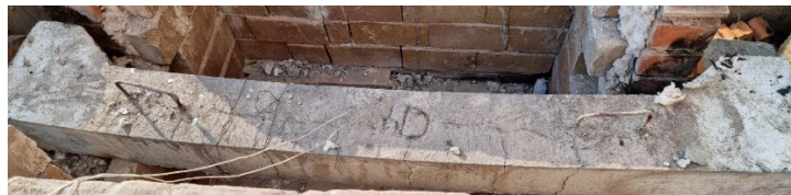
(c) Crack pattern for 750 °C temp. Specimen.
